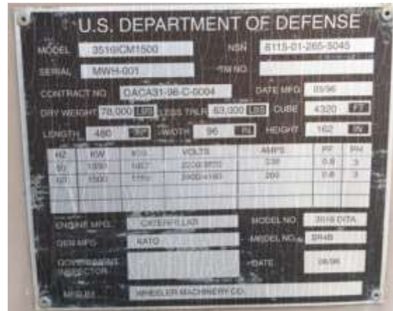
Generator Set Nameplate
